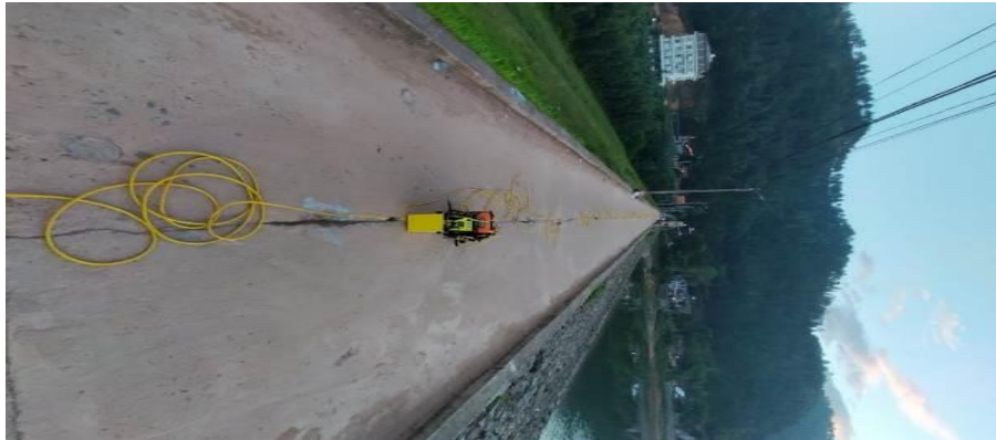
Figure 1. Current status at the top surface of the Dong Do dam
